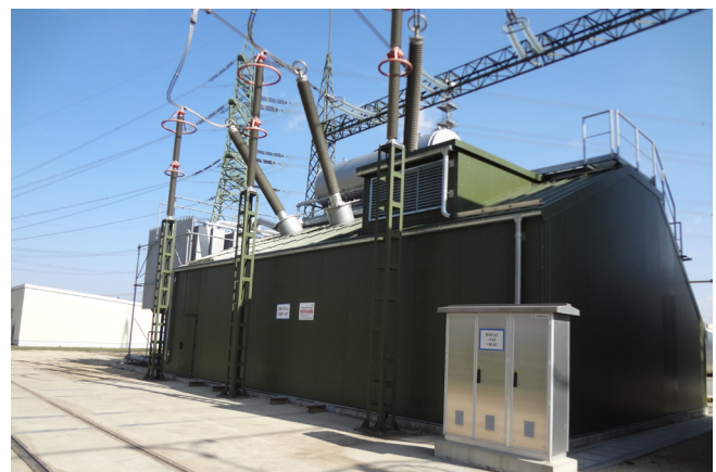
Power transformer with sound house
