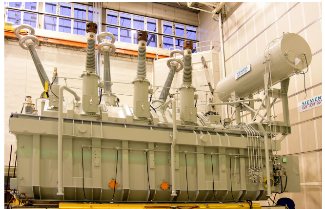
Transformer in the extra-high voltage test hall
