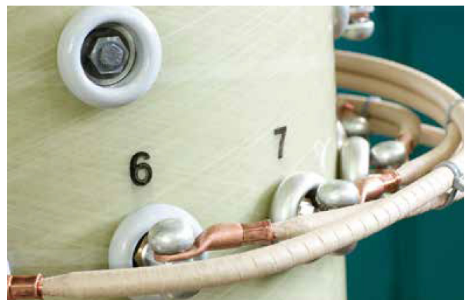
On-load and deenergized tap changers ensure that the output voltage remains constant
