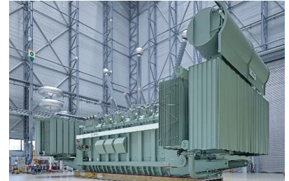
Transformer 420 kV/ 400 MVA Power Transformer
