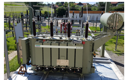
Transformer 31,5/40 MVA, 112/20 kV Power Transformer
