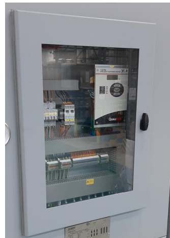
Image 6-13: Control cabinet in enclosure
