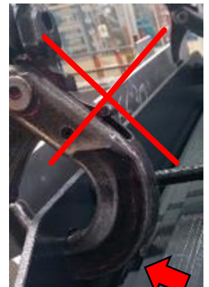
Image 5-6: Crane hook rests on upper yoke
