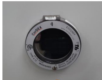
Image 6-20: Infrared window on the transformer enclosure
