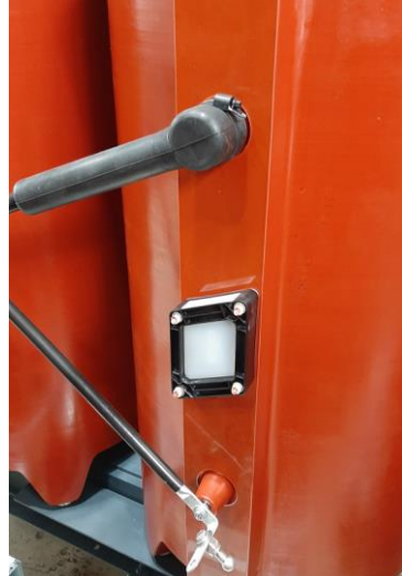
Image 5-25: Covers on switch tubes and HV taps
