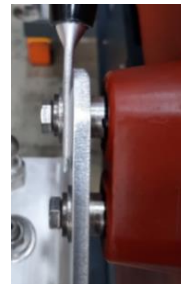
Image 5-26: Arrangement of the washers on switch tubes on the HV connection
