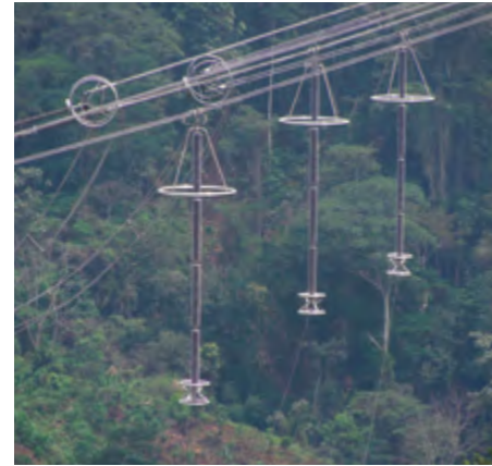
550 kV line in Colombia NGLA solution realized with 3EL2
