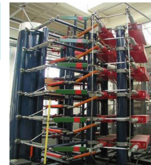
Test generator supplying both impulse voltages (1.2/50 μs and 250/250 μs) and impulse currents (8/20 μs and 30/60 μs)
