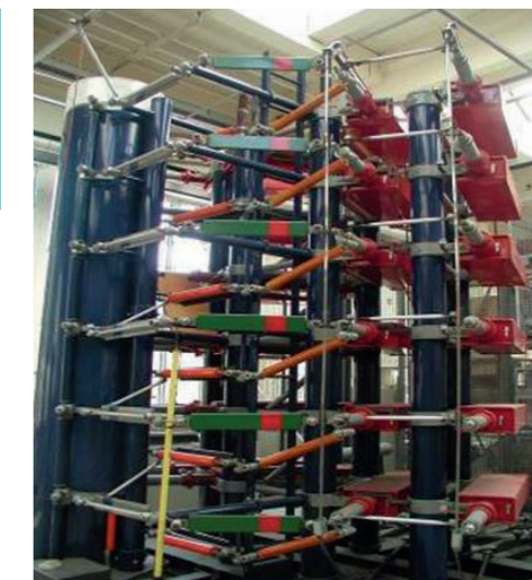
Test generator supplying both impulse voltages (1.2/50 μs and 250/250 μs) and impulse currents (8/20 μs and 30/60 μs)
